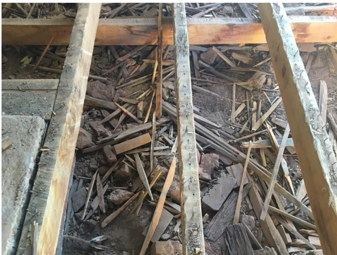
Main building waiting room waste material found under sub-flooring
