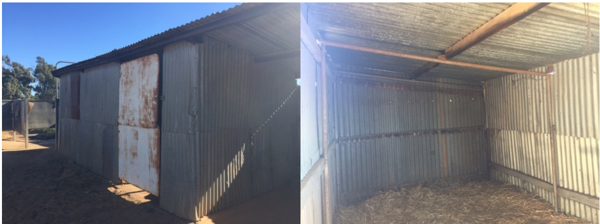
Existing Swabbing Shed
