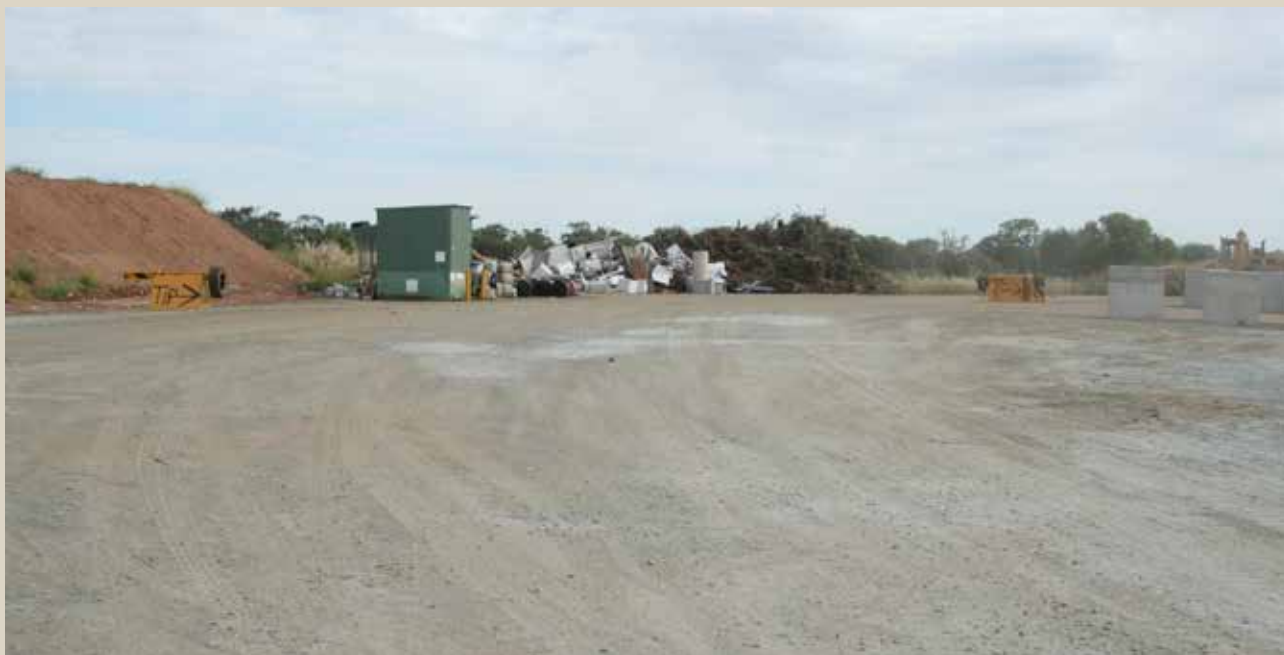
Nyngan Waste and Resource Recovery Facility Levelling of Existing Site for Recycling Drop off Area, February 2016
